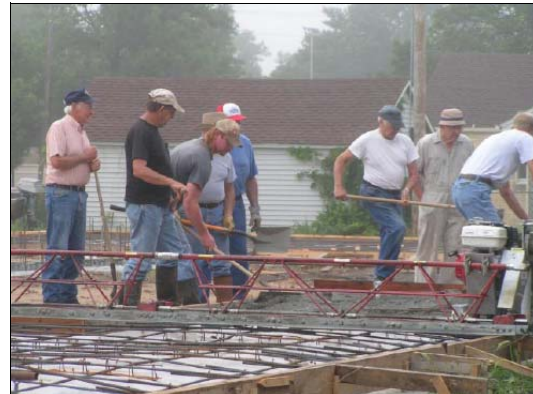
Volunteers work together to pour concrete for the Glasco KAN STEP Fire Station project. Courtesy photo by Lynne Imboden, Glasco City Clerk.
