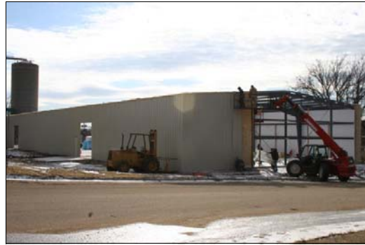
Construction took place this Spring on a new building that will house business operations of M & G Designs, Inc. in Sylvan Grove.
