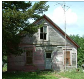
Many communities have at least one dilapidated property such as the one above. This structure has since been demolished with assistance from a CDBG grant.
