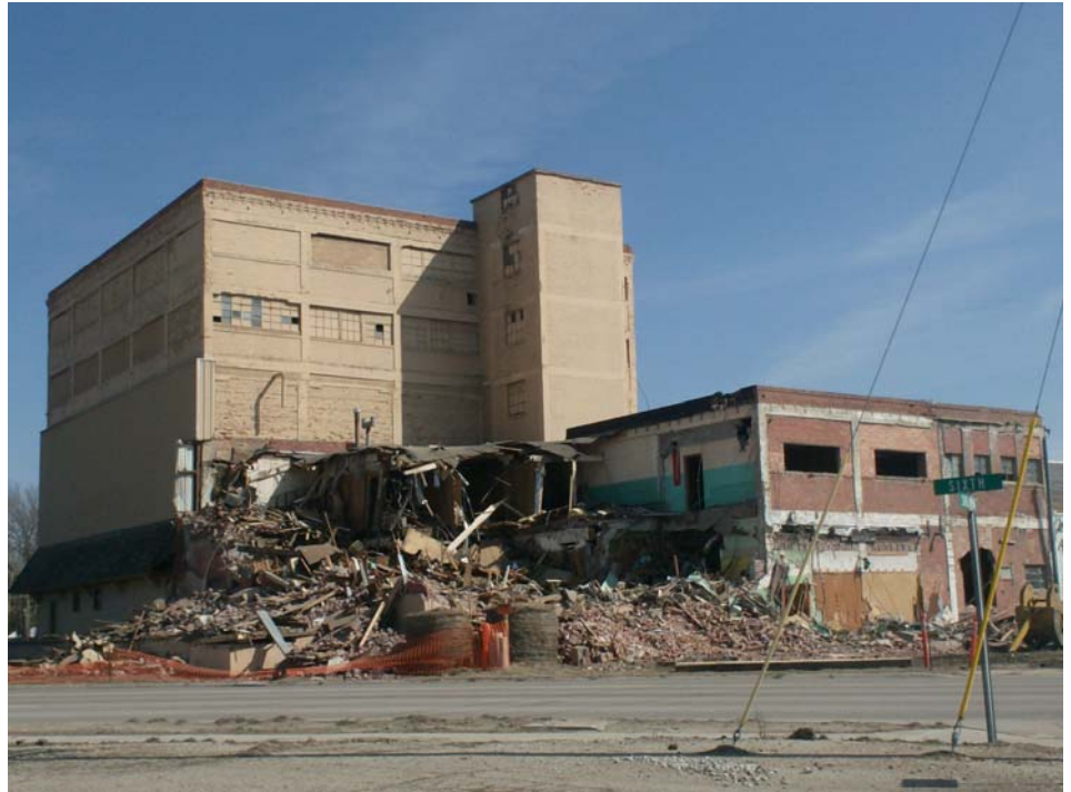
The Swift Building in Clay Center was demolished, which cleared the way for GT Manufacturing, Inc. to expand and add more employees.
