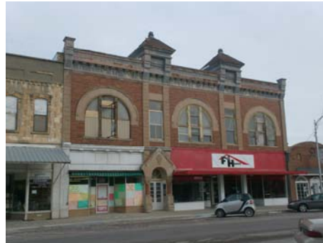
This retail structure located at 111-115 East Main in downtown Beloit will be stabilized and repaired with the help of funding from the recent CDBG award.
