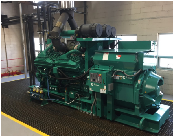
A new generator has improved the reliability of the power supply in the City of Lincoln Center.
